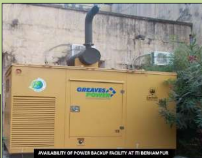
Power Back Up Facility
